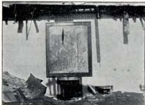
COURT ROOM AFTER THE FIRE.
